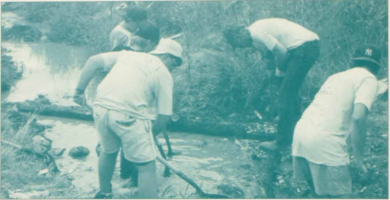
Volunteers at work on Oregon's Bridge Creek adding to channel structure and complexity (photo by Hugh Barrett).
